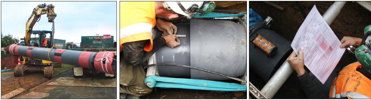
FIG. 14 Typical handling, jointing and workmanship quality checks of DN400 Kurimoto SRDIP installed at Cleat Street Porirua City, New Zealand.
