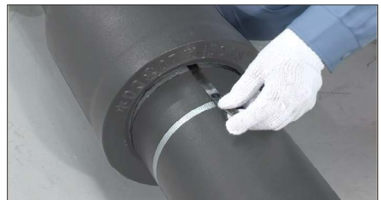
FIG. 13 Quality assurance check with an installed pipe-joint measuring the pipes gasket position to the first witness mark.
